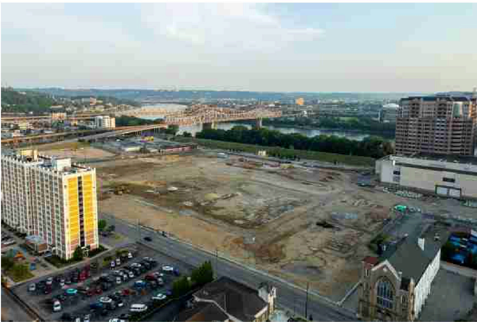
Excavation work was underway this summer at the Covington Central Riverfront site in downtown Covington, Ky.
